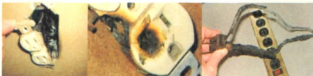
图 7 因接触电阻和过负荷造成的线路烧毁故障实例 Fig. 7 Fault example of the circuit burning due to contact resistance and overload
