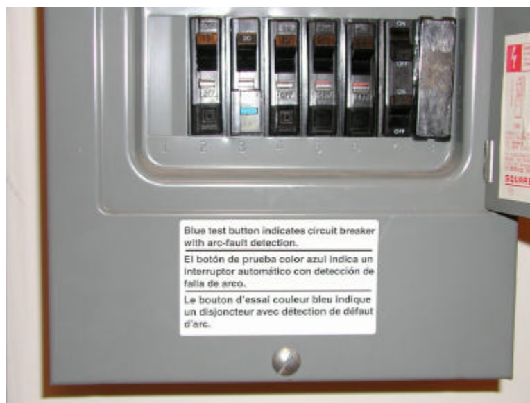
Figure 5 – AFCI breaker (2nd from left) and Test Button Label
